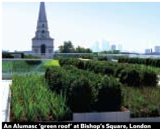
An Alumasc 'green roof' at Bishop's Square, London
